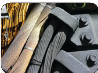
Air cooled connections
